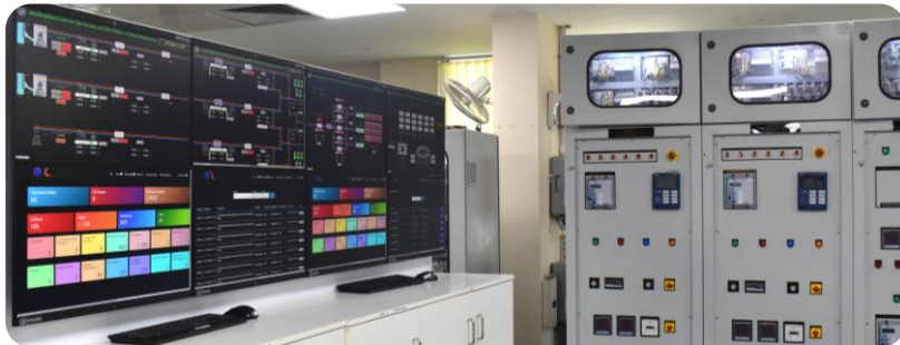
OT SOC & SCADA with Power Hardware-in-the-loop (PHIL) Test Bed
